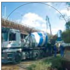
Ready-mixed concrete plants
